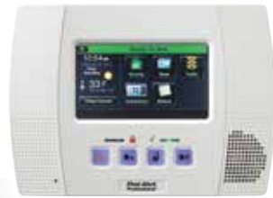
Keypad with Combination Panel & Home Automation Controller
